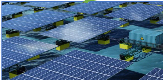
SolarinBlue France 2020 50 kWp per floater
